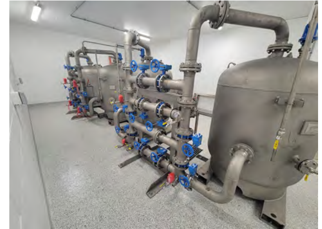
PFAS Treatment at Avon Well 3
